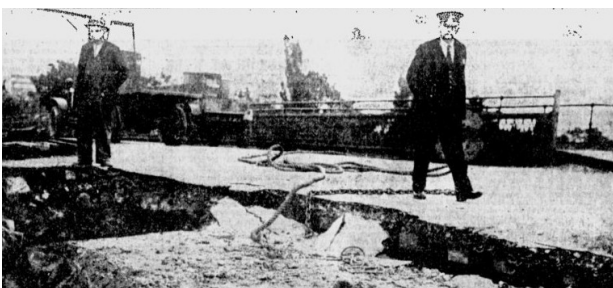
Damage to the road surface on the Richmond side of the Wallen Road Bridge - 3 December 1934. Photo from The Age newspaper.
