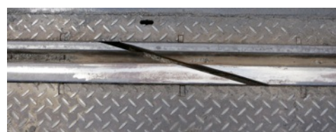
Diagonal gap separating each rail in the centre of the bridge. Photo: Ed
