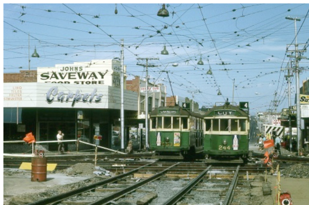
W3 659 and W2 244 pass at South Caulfield Junction during relaying work in 1966. The connections at the junction were changed at this time, and the tangle of overhead wires shows remnants of abandoned curves.
