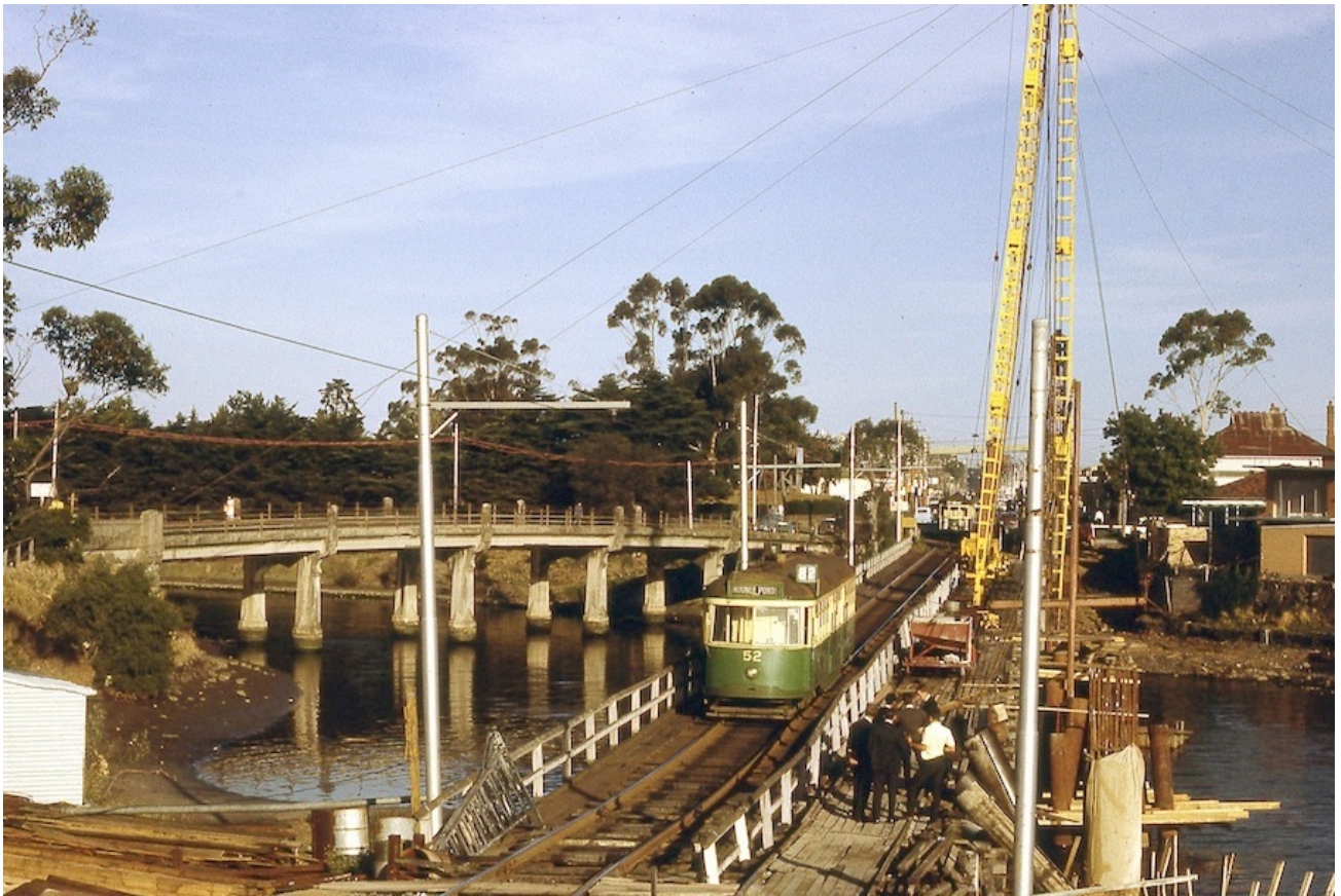
Work is under way on the new bridge over the Maribyrnong River, and the tram line has been reduced to single track as VR 52 heads for Moonee Ponds in 1966. Photo: Dale Budd
