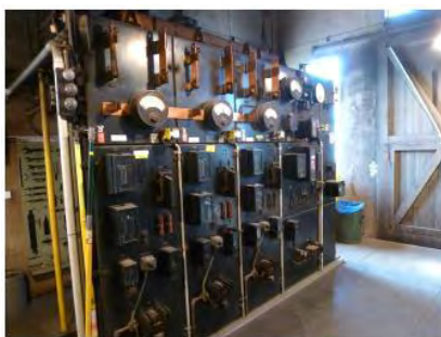
ABOVE: Open panel switchboard inside Brunswick West (2019).
