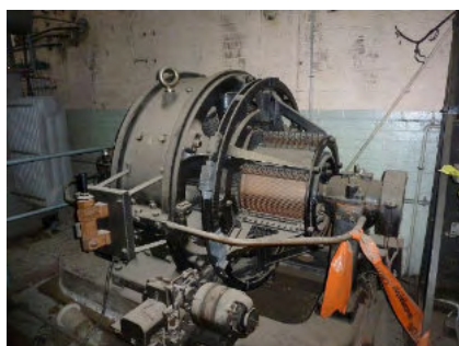
BELOW: Decommissioned rotary converter inside the Brunswick Rd Substation (2019).
