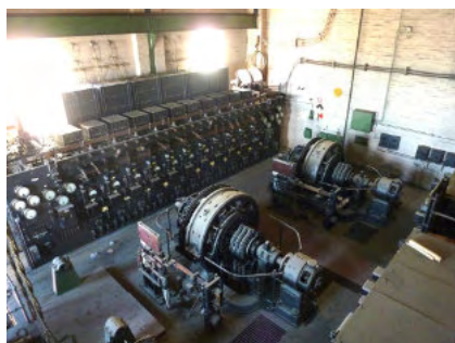
ABOVE: Two rotary converters and the open panel switchboard inside the decommissioned Malvern Tram Depot Substation (2019)
