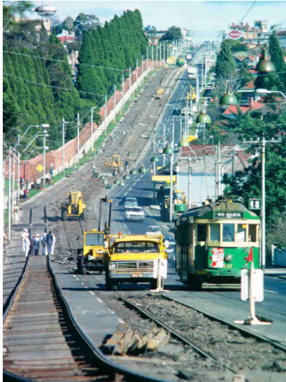
ABOVE: W2 class 532 bound for North Balwyn passing trackwork on High St, Kew (1978).
