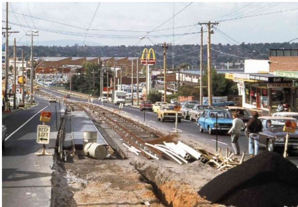
ABOVE: Track laying in Burwood Highway looking east from Warrigal Road toward Evans Street (April 1978). Note the trolley wire already in place.
