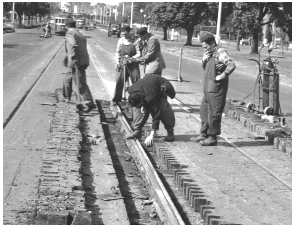
Neatly stacking wooden blocks was a key skill of Melbourne's tram track repair crew in 1953. Photograph from the collection of the Melbourne Tram Museum.
