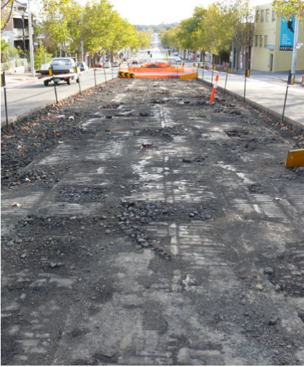
Woodblocked cable tram tracks uncovered during road works in Abbotsford Street, North Melbourne in 2007, 72 years after they last carried trams. Photograph by Russell Jones.
